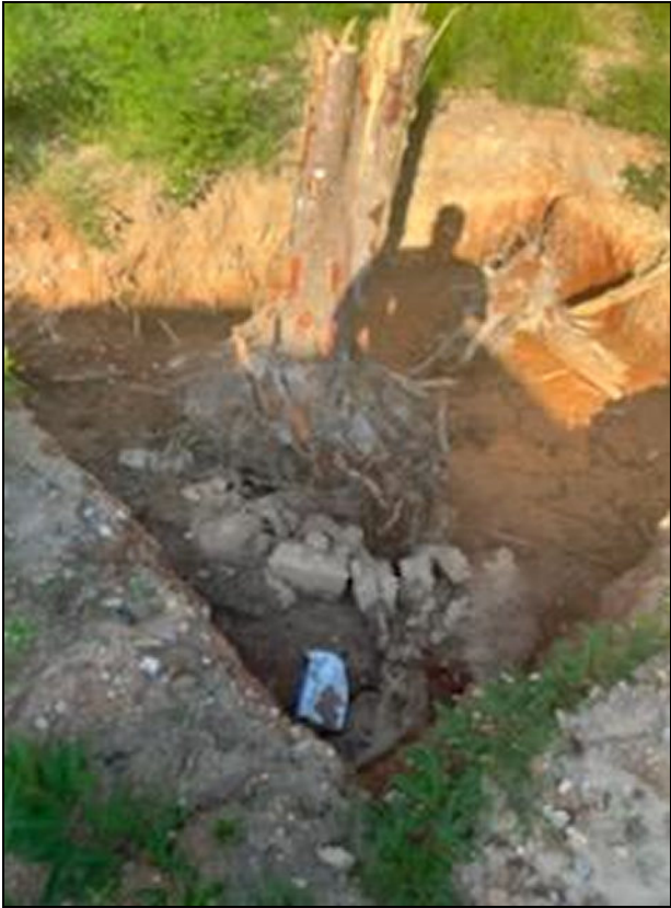
Photos of buried debris areas near accessory building
