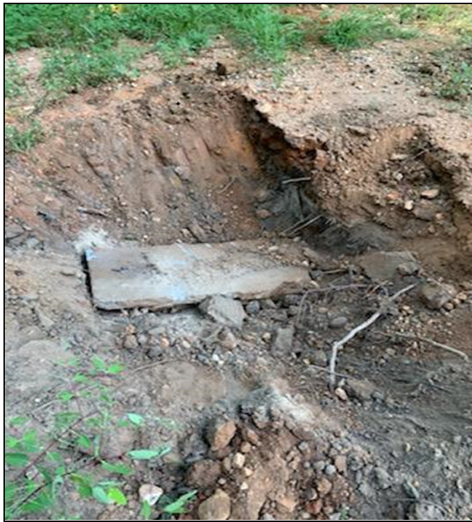
Photos of buried debris areas near accessory building
